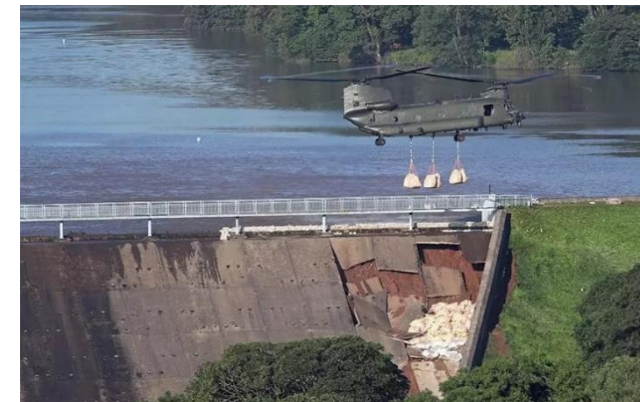
Whaley bridge Dam, Danny Lawson/PA 2019
